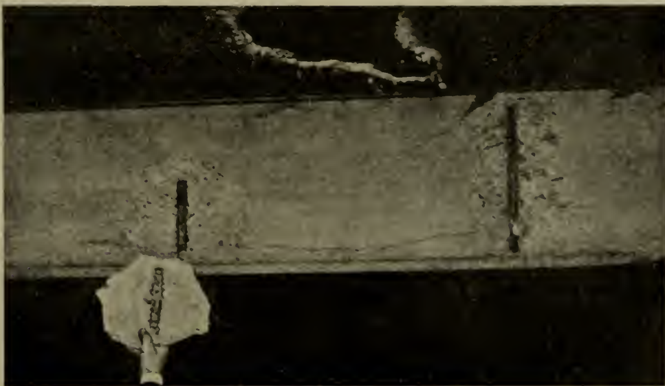
FIG. 9. ELECTROLYTIC CORROSION OF STEEL REINFORCEMENT: CONCRETE FORCED OFF STIRRUPS OF BEAM.
